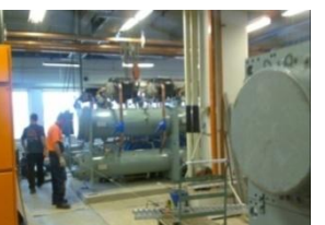
One of the RBA chillers
