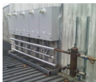
Mitcham 150 kw Heating System
